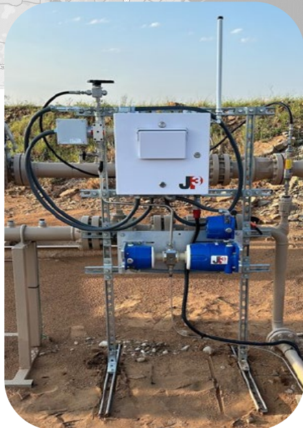
No Shelter, No Calibration Gas, Remotely/Continuously Monitored
