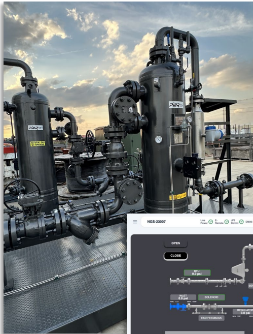
Smart Filtration Skid
