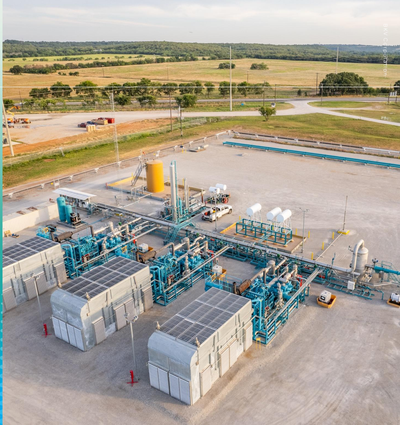
Barnett Zero compressor facility Wise County, Texas
